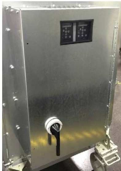
Figure 4. VFD per fan (outside)
