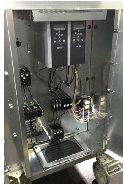
Figure 5. VFD per fan (inside)
